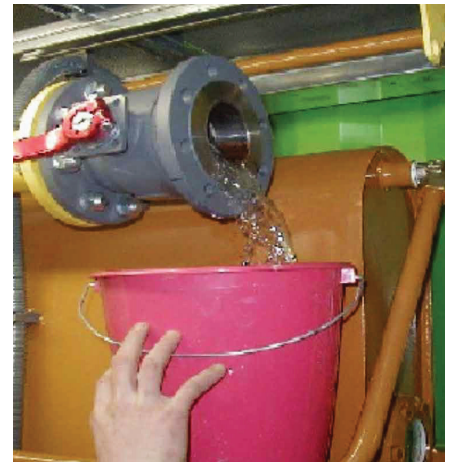
Fig 1 – Water condensate in biogas pipework
