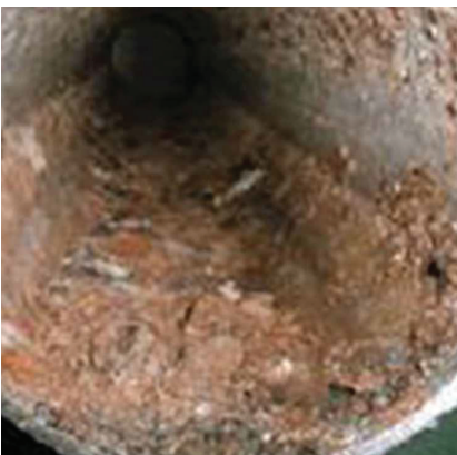
Fig 2 – Corrosion in storage vessel
